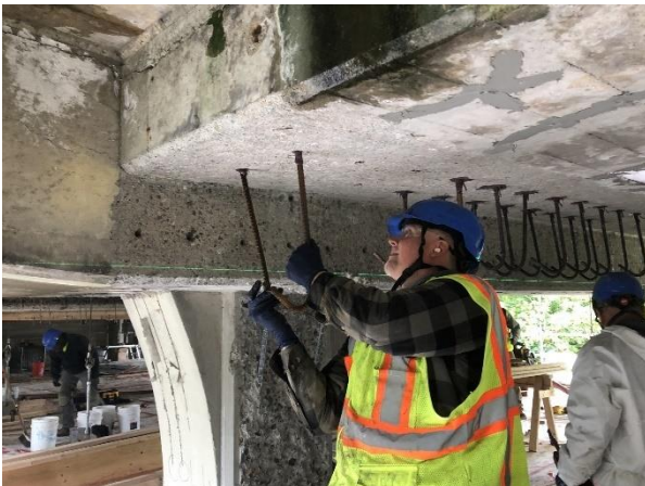
Installing pieces of metal called rebar under the McGraw St Bridge. This rebar will later be embedded inside of concrete to increase its strength.
