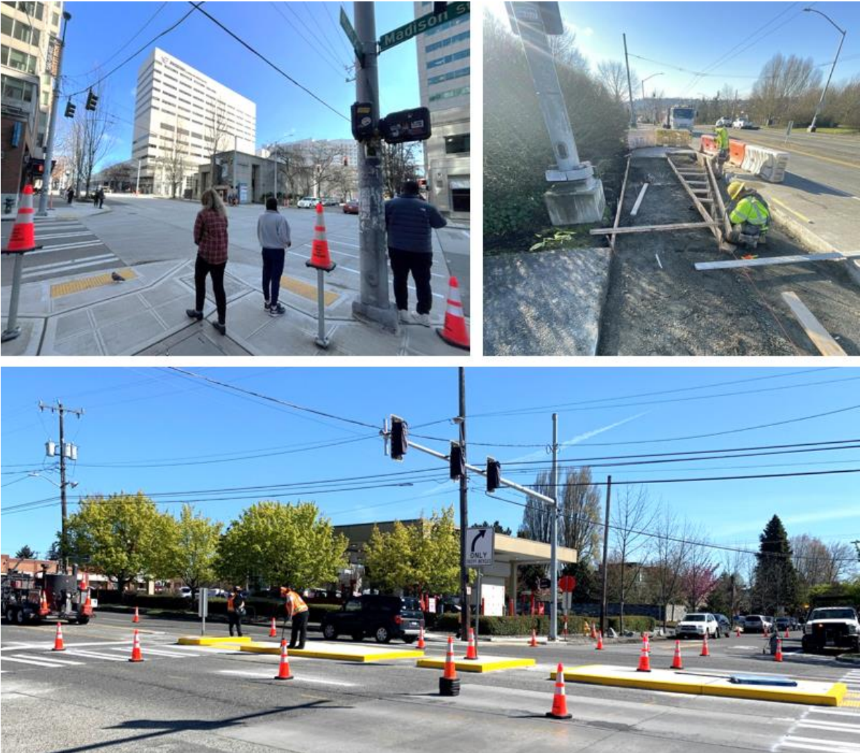
Construction is in full swing on many projects. Clockwise from top left: new curb ramps and crossings on Madison St, installing a new sidewalk as part of the MLK Jr Way S Safety Project, and a new crossing and signal as part of the 15th Ave NW & NW 83rd St Pedestrian Safety Enhancements Neighborhood Street Fund project.
